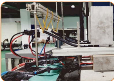
Temperature rise test
